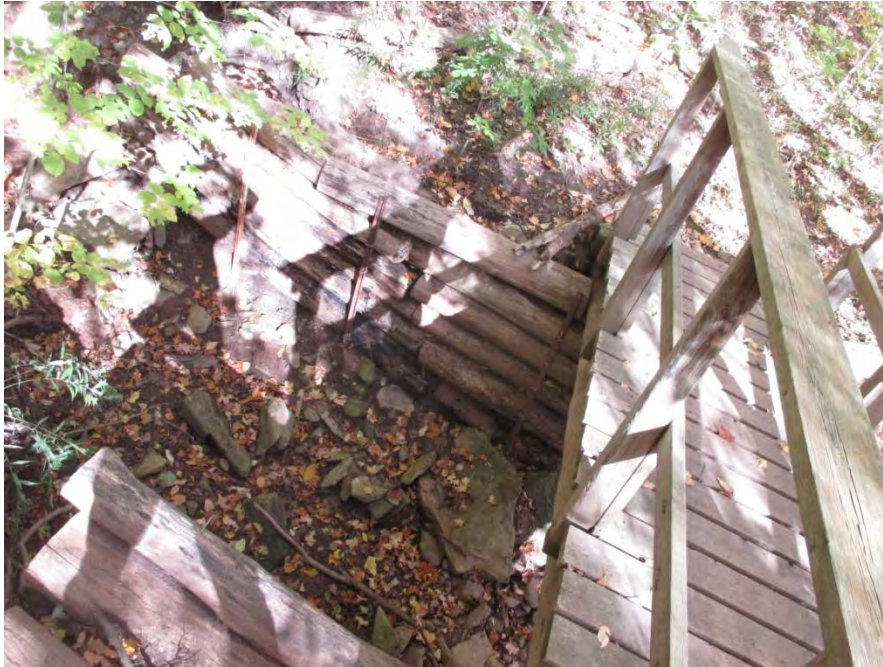
Photograph 11: Creek erosion and bank failure at bridge located on Bruce Trail.
