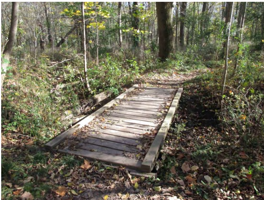
Photograph 2: Failing/undersized bridge structure on Ray Lowes Side Trail.
