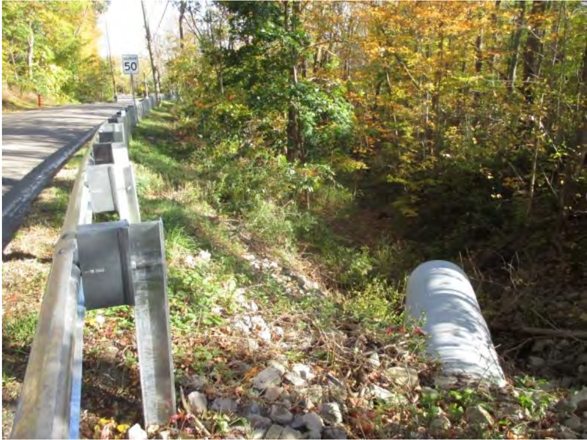
Photograph 8: Perched outfall at edge of Borer's Falls Conservation Area 1, near Valley Road.
