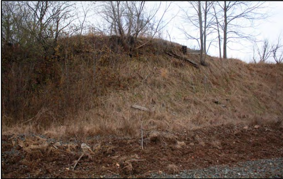
Photograph 1: Remnant earthen abutments of former bridge over railway tracks at Hopkins Tract. Facing northwest. Photograph courtesy of Nigel Finney, Conservation Halton.
