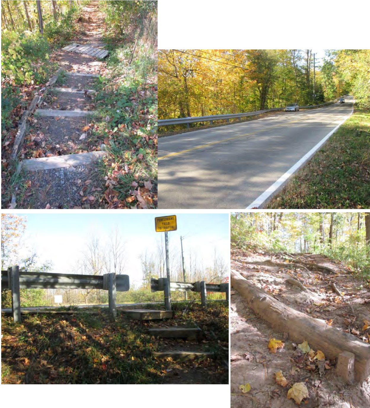
Photograph 9: Entrance to Bruce Trail on west side of Valley Road. Steep earthen staircase in poor repair. Parking pull-off on Valley Road.
