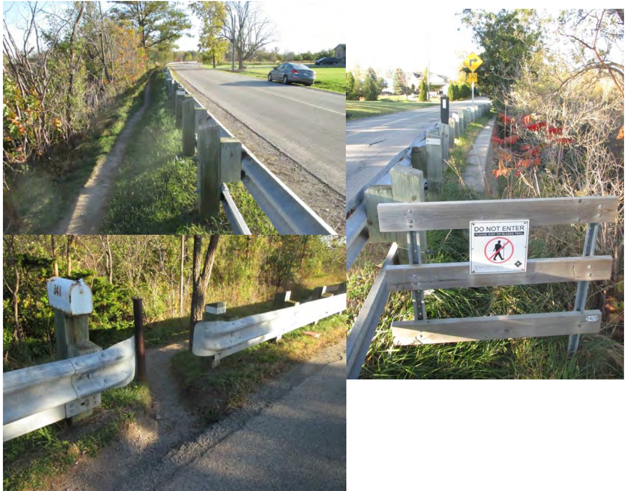
Photograph 21: Bruce Trail along Rock Chapel Road passes through gaps in the guardrail. Hikers must walk off the road behind the guardrail for a section, and then on the road for a section. The section of trail behind the guardrail is along the top of a steep cliff.
