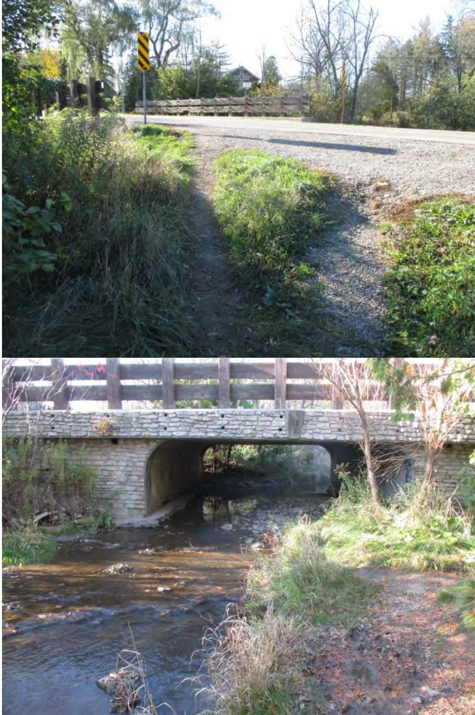
Photograph 20: Access to Bruce Trail from Rock Chapel Road into Rock Chapel 4. Hikers must hike along the road and cross the bridge to access the Bruce Trail. Unsanctioned trails leading to the creek.
