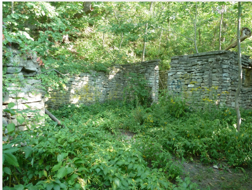
Photograph 1. Dry stonewall ruin located along Bruce Trail in Little Property (taken by Leah Lefler).
